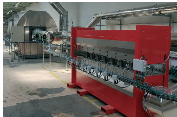
Power to heat
