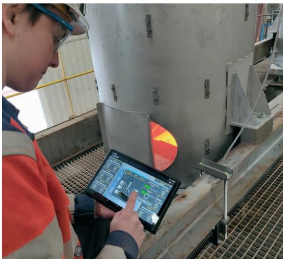
Tests during the commissioning of a high-temperature fume collection system on one of the tiling kilns and validation of the command control and mechanical systems, Pontigny site.
